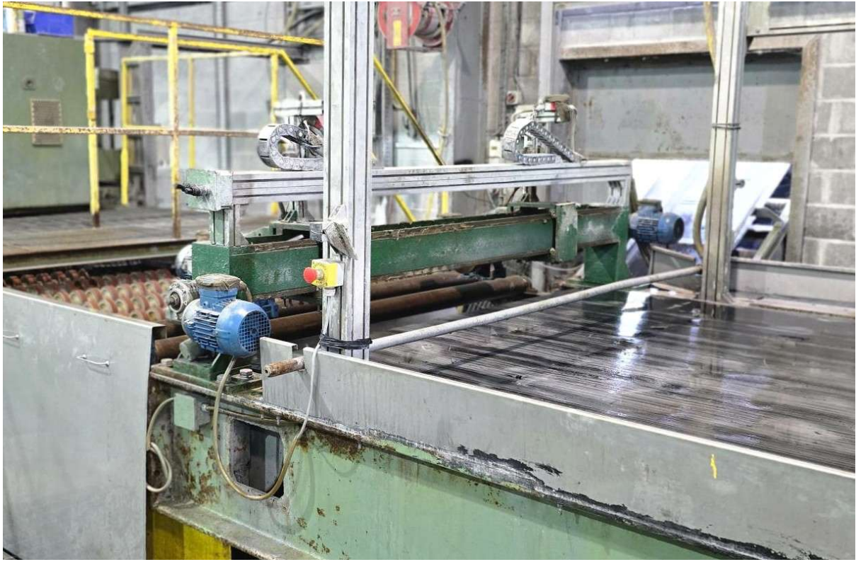
Waste Breaker and Waste Conveyor
